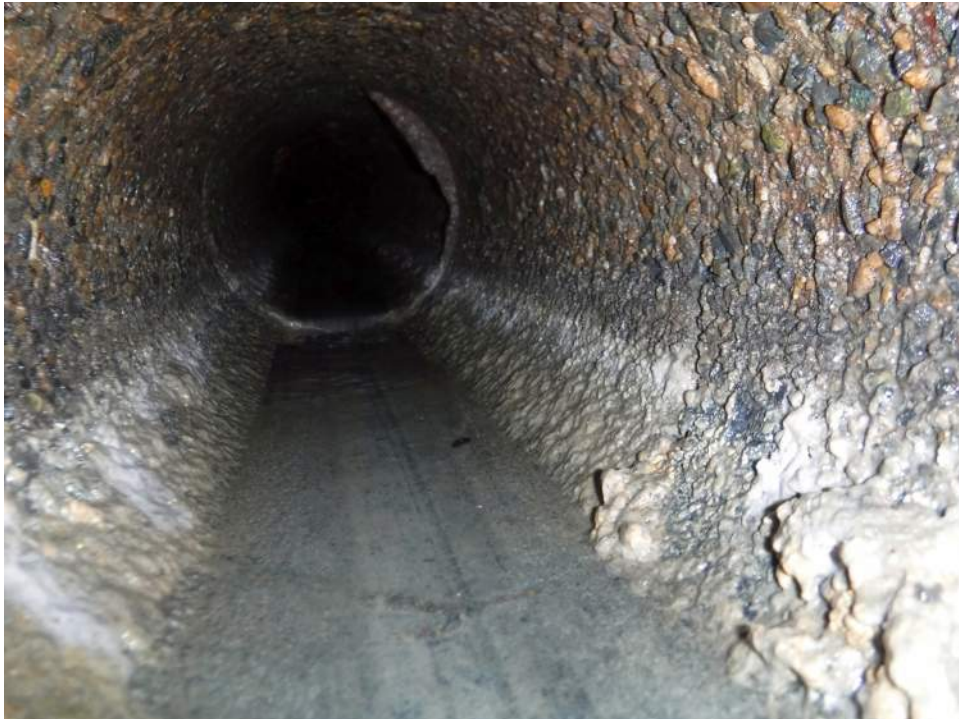
Southwest Influent Pipe
