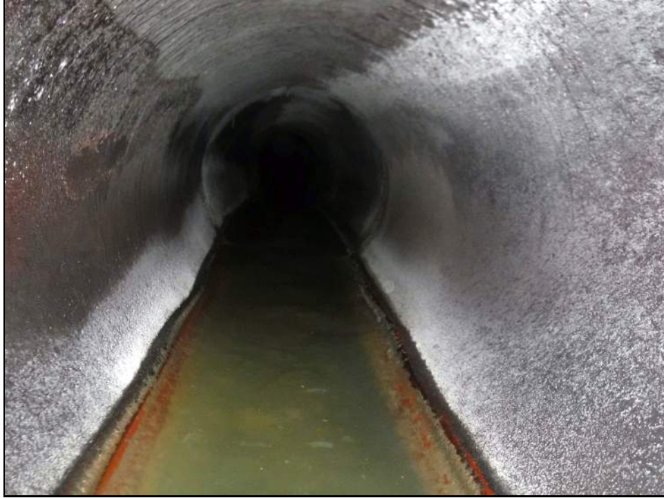
Mounted Northeast Influent Pipe
