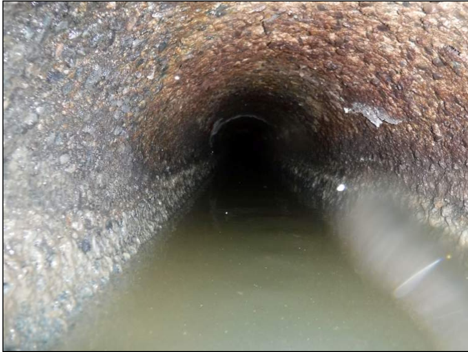
North Influent Pipe
