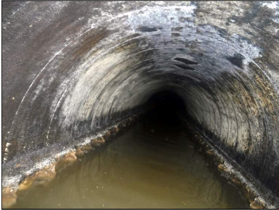
North Influent Pipe
