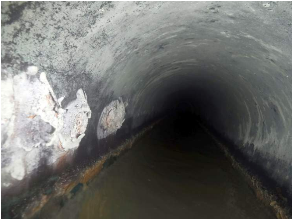
Mounted Northwest Influent Pipe
