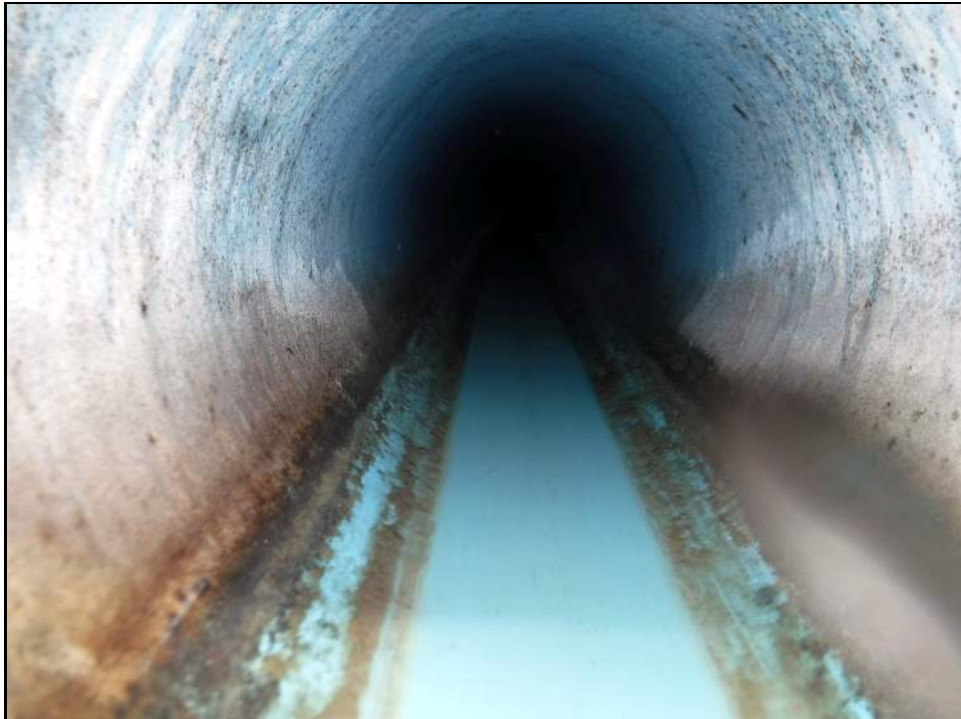
Mounted Northeast Influent Pipe
