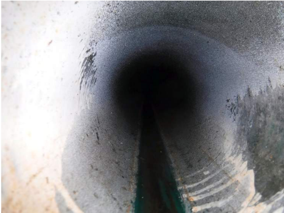
Northwest Influent Pipe
