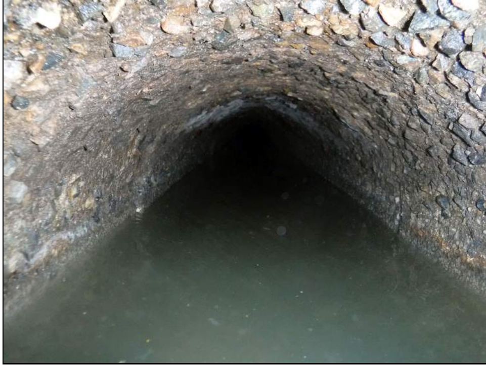
Mounted Northeast Influent Pipe
