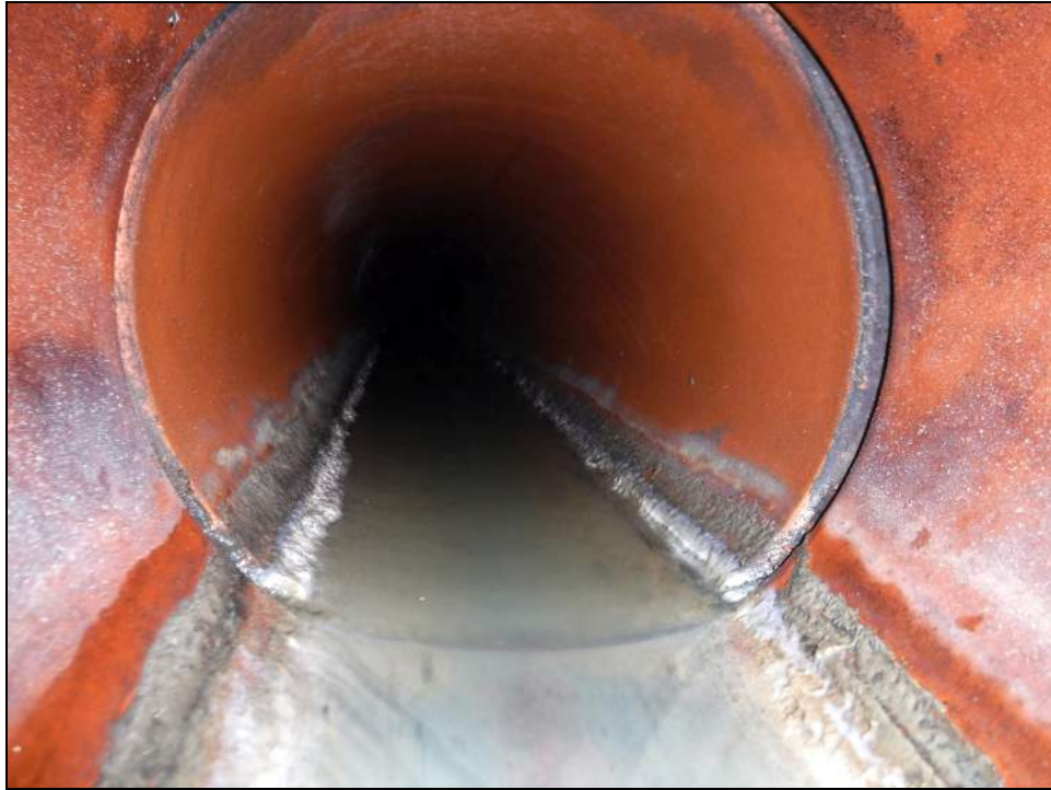
Mounted Northeast Influent Pipe
