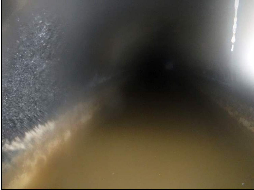
Mounted North Influent Pipe
