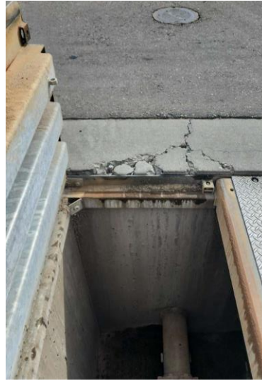
Photo 7-18 Site / Civil – Concrete cracks next to pump discharge piping vault, minor spalling, rusted lid bolts
