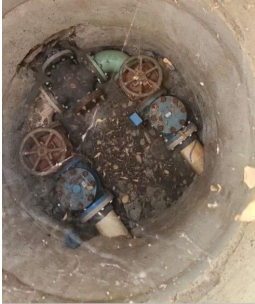
Photo 7-29 Mechanical – Check valve from original plant
