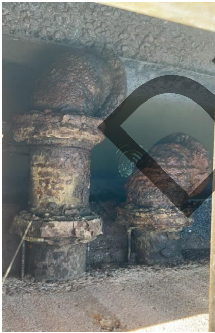
Photo 7-3: Mechanical – Worn pump discharge piping
