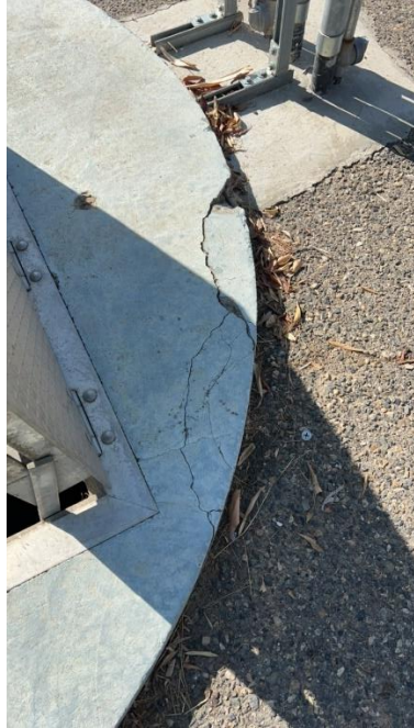
Photo 7-5: Site / Civil – Cracks on concrete next to wet well cover
