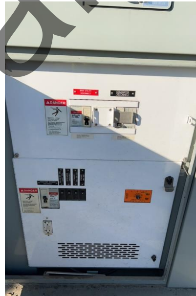
Photo 7-28 Electrical – Meter/Main Panel
