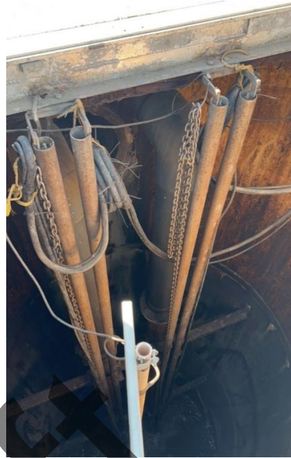
Photo 7-6: Structural / Architectural – Minor corrosion on guide rails
