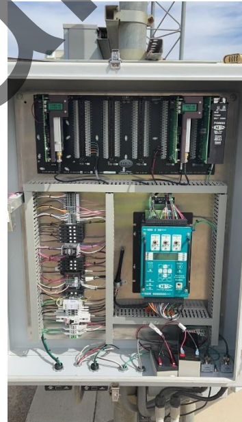
Photo 7-16 Electrical & Power – Power panel installed last year
