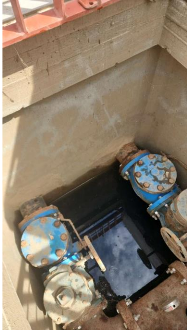
Photo 7-13 Site / Civil – Standing water in pump discharge piping vault
