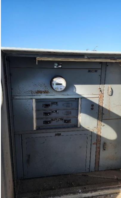
Photo 7-1: Electrical & Power – Main Breaker not Upgraded in 2023
