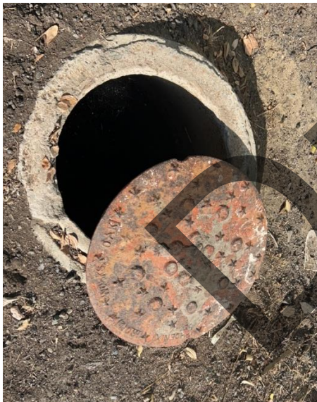
Photo 7-31 Site / Civil – Pump discharge piping vault, planning on putting in new vault
