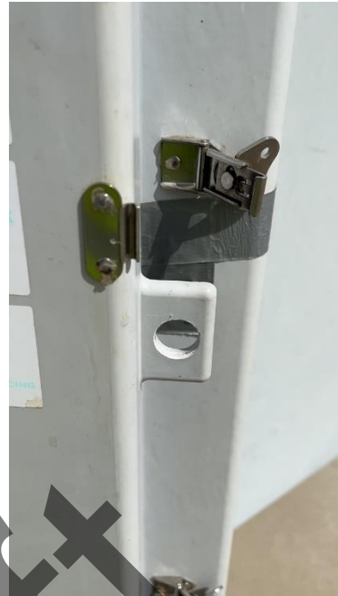
Photo 7-14 Electrical & Power – Broken hasp on power panel
