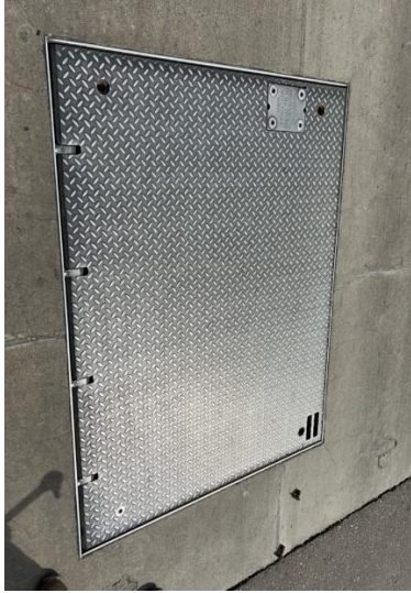
Photo 7-17 Site / Civil – Handle missing on wet well cover
