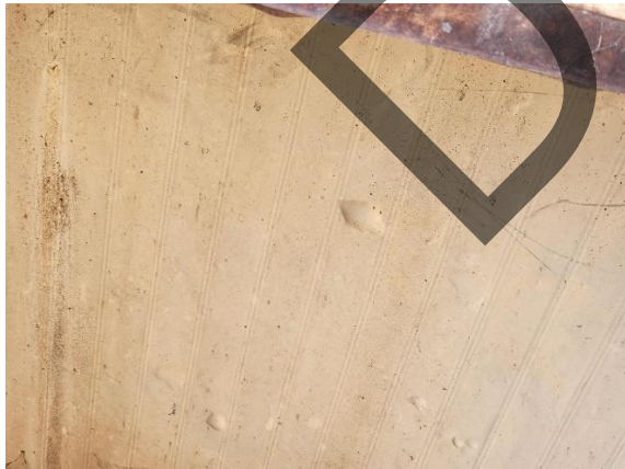
Photo 7-11 Mechanical – Minor bubbling on wet well t-lock
