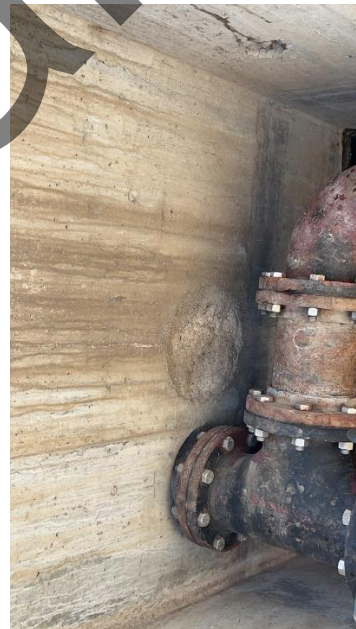
Photo 7-12 Site / Civil – Minor cracks, voids, and spalling in pump discharge piping concrete vault
