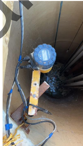
Photo 7-24 Electrical – Ultrasonic level transducer
