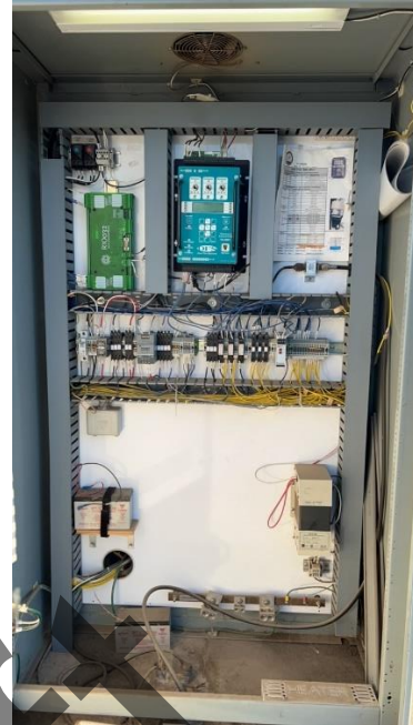
Photo 7-22 Electrical & Power – PLC panel rehabilitated in 2012
