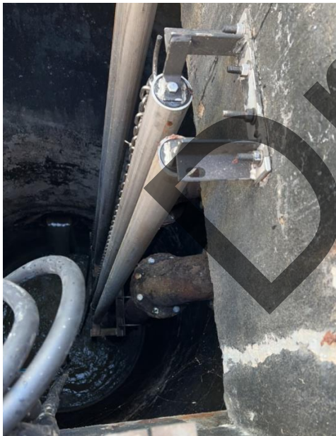
Photo 7-35 Mechanical – Corrosion on discharge piping
