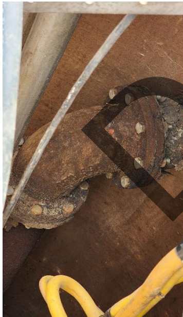
Photo 7-15 Mechanical – Corrosion on pump discharge piping
