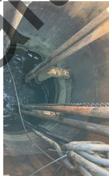
Photo 7-32 Mechanical – Corrosion on guide rails
