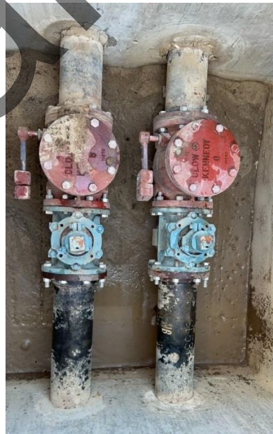
Photo 7-36 Site / Civil – Sand buildup in discharge piping vault
