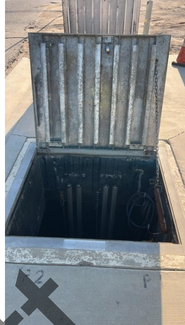
Photo 7-34 Site / Civil – Worn lid and safety cover for wet well
