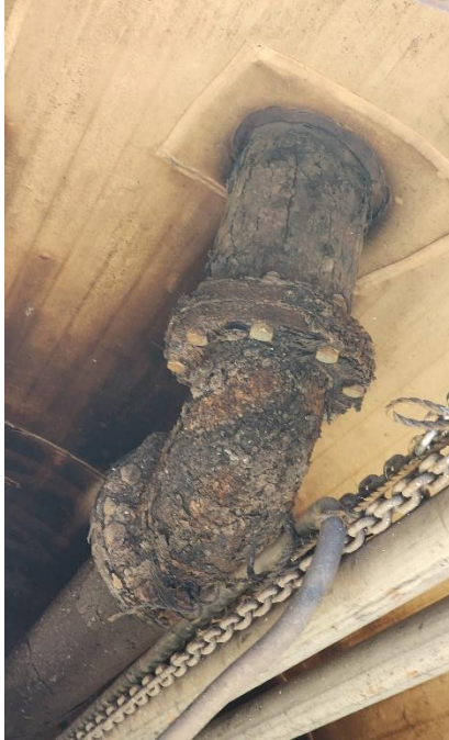
Photo 7-9 Mechanical – Corrosion on Discharge Piping
