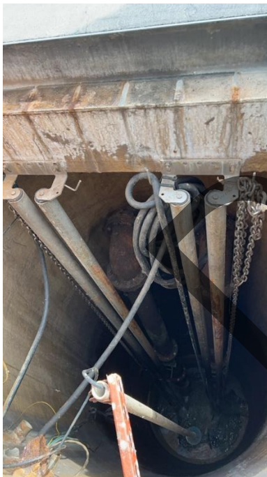
Photo 7-19 Structural / Architectural – Corrosion on guide rails
