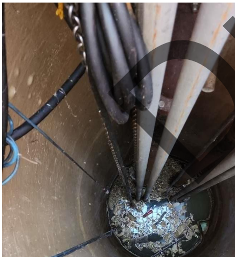
Photo 7-23 Structural / Architectural – Minor bubbling on wet well
