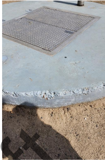
Photo 7-10 Site / Civil – Minor cracks and spalling along top of wet well
