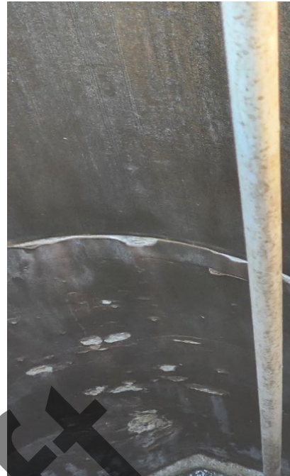
Photo 7-2: Site / Civil – Wet well t-lock liner pulling away
