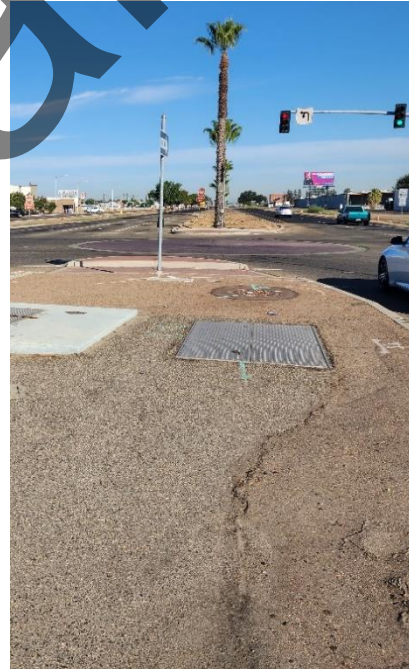
Photo 7-4: Structural / Architectural – Cracks on asphalt near pump discharge piping vault
