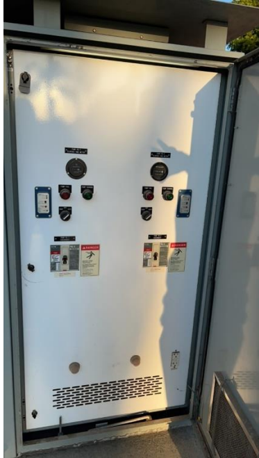
Photo 7-21 Electrical & Power – Control panel rehabilitated in 2012
